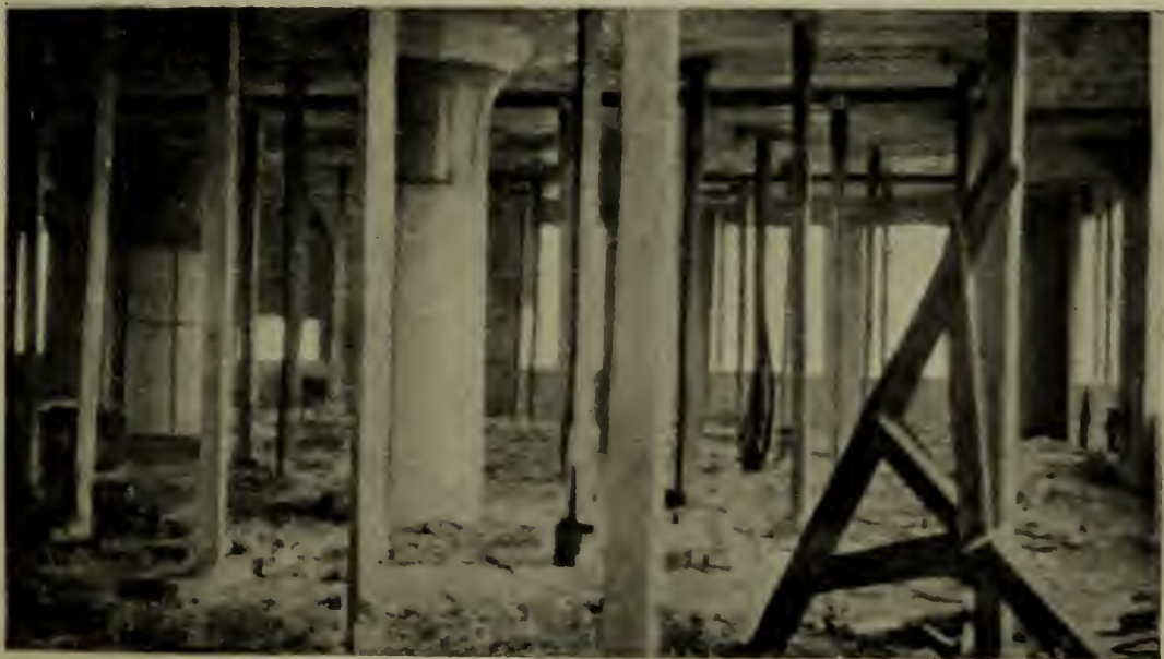
FIG. 5. METHOD OF SHORING SLAB AFTER ALL BUT ONE ROW OF METAL SLAB FORMS HAVE BEEN REMOVED.
